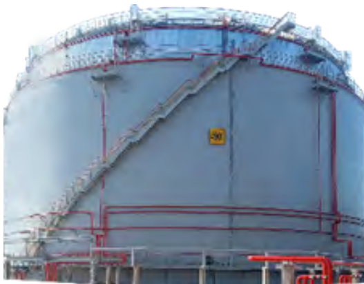
Vertical steel tank with protective wall or 'double wall storage tank' (PBC3C)
