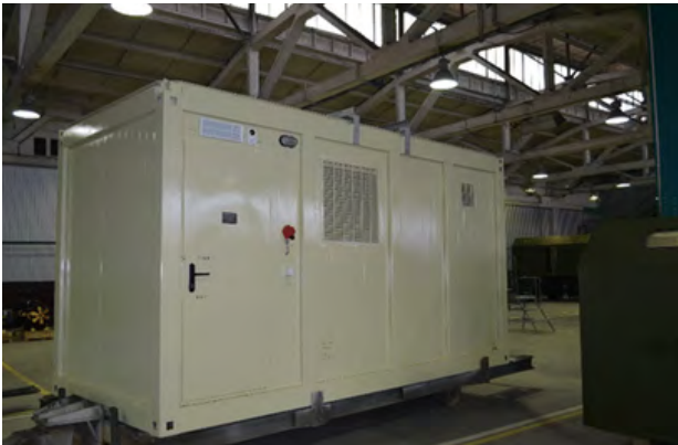
Diesel power plant
