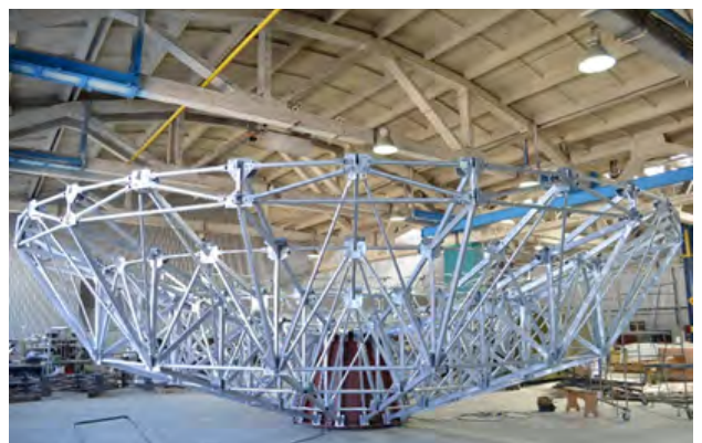
Antenna system components
